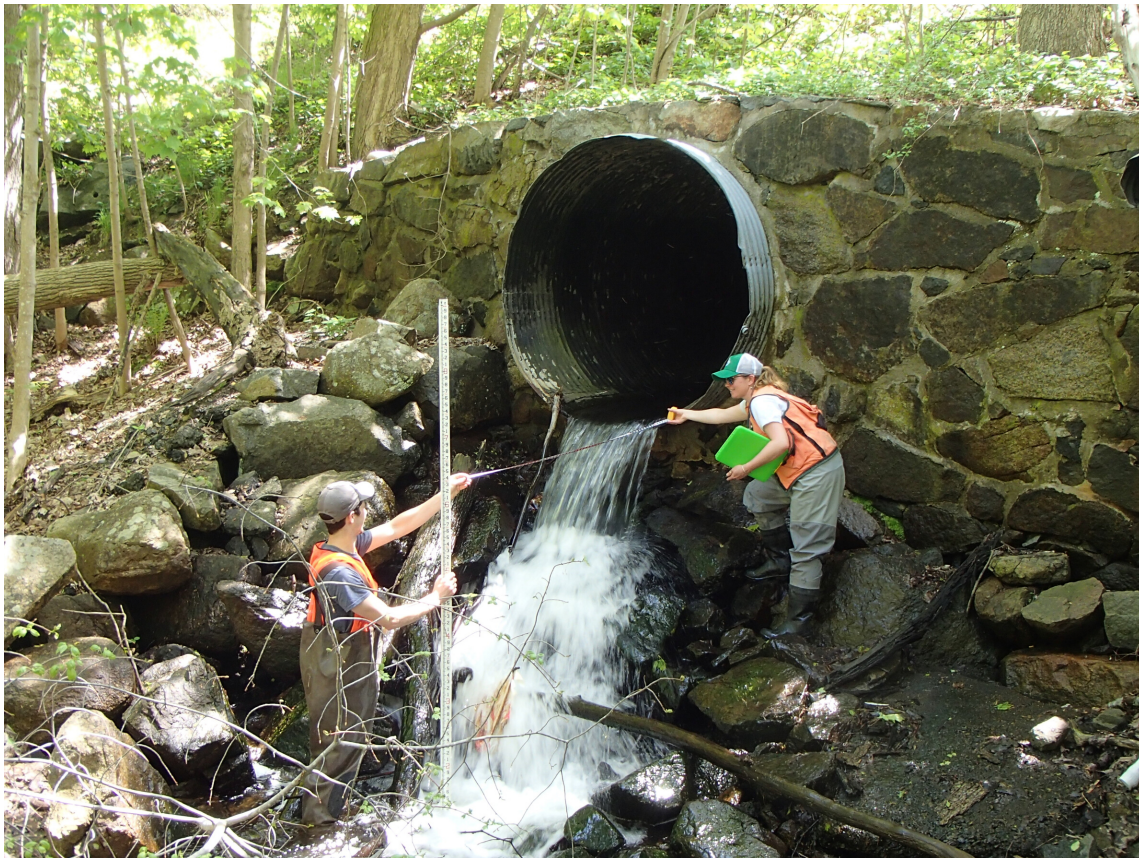
Jacob Lehan of the Division of Ecological Restoration and Kaitlyn Shaw measure the outlet drop of a severely perched culvert in Gloucester.
