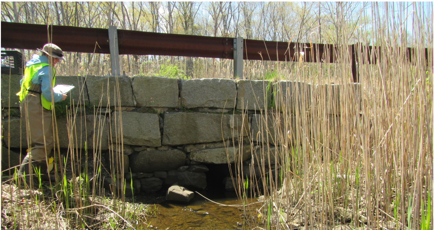
Stream crossing field technician Kristen Thiebeault assesses an undersized stone crossing.
