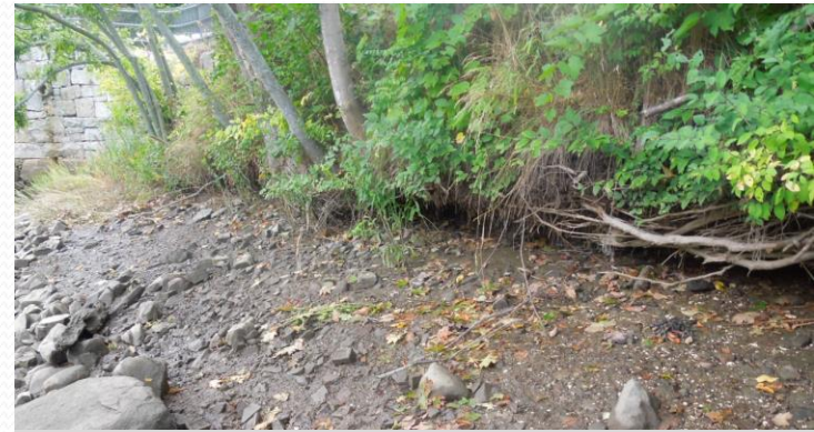
Erosion (undercutting) of coastal bank on Water Street
