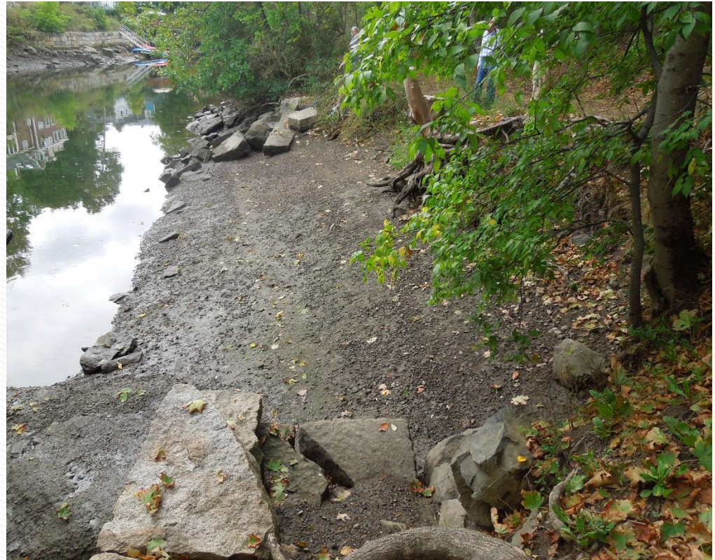
Erosion of an unarmored area between a seawall and a revetment by the Green Street Bridge
