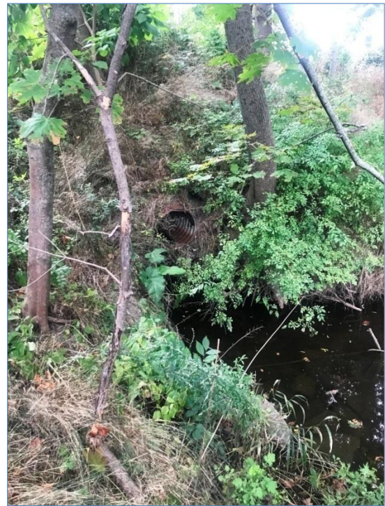
Photo 1. View of 18-inch corrugated metal pipe that discharges stormwater into the Ipswich River at the site along County Street. The land beneath the culvert is deeply undercut.
