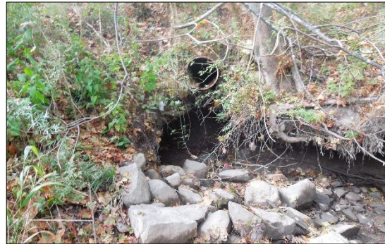
Significant erosion of river bank from failed stormwater culvert near County Street and Shurcliff Riverwalk.
