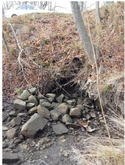
Image #3: Area 4 – Eroded Bank at Outfall
